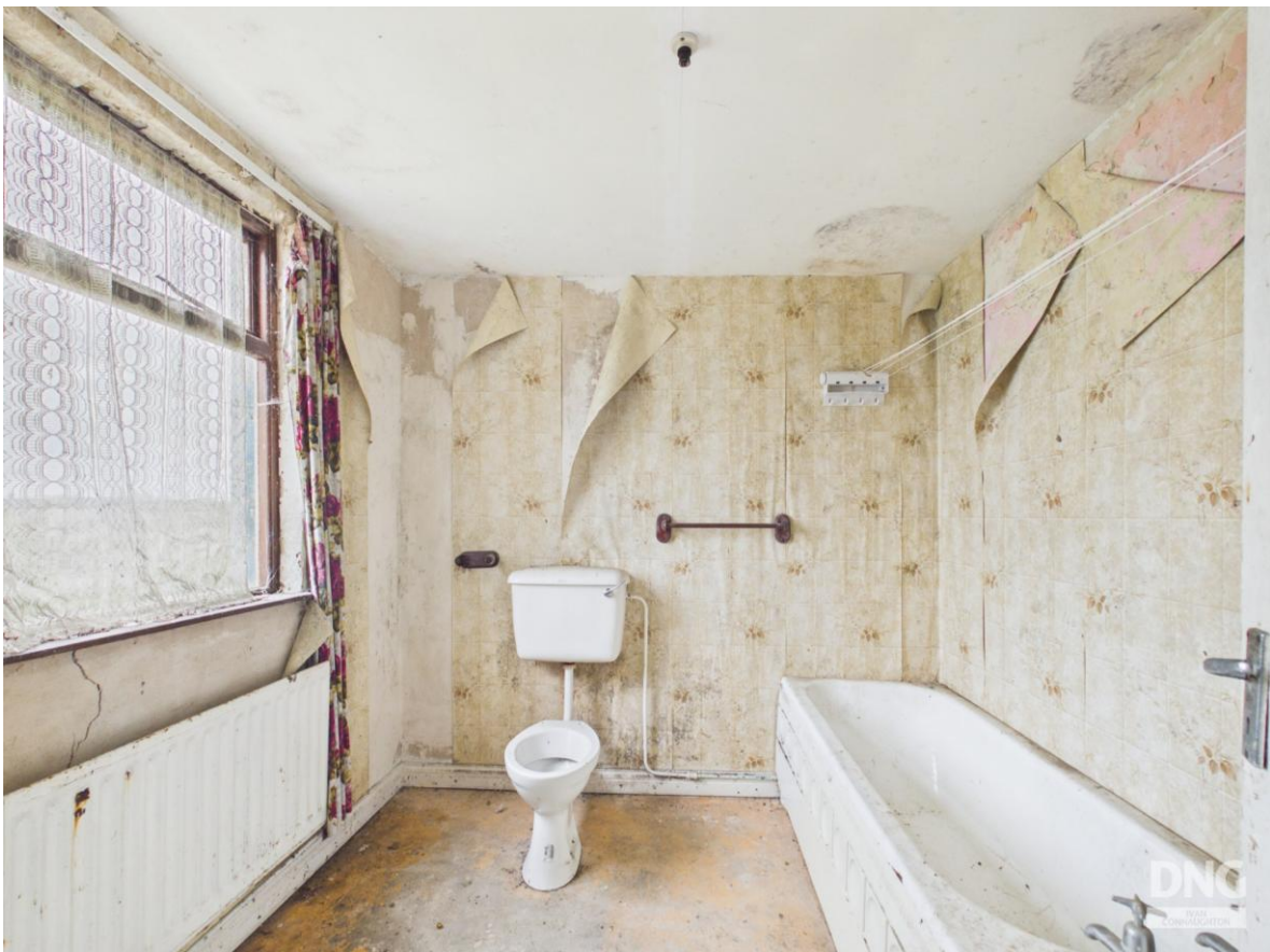
Derelict Residence, Ashbrook, Strokestown, Co. Roscommon
