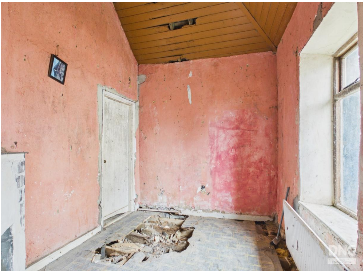
Derelict Residence, Ashbrook, Strokestown, Co. Roscommon
