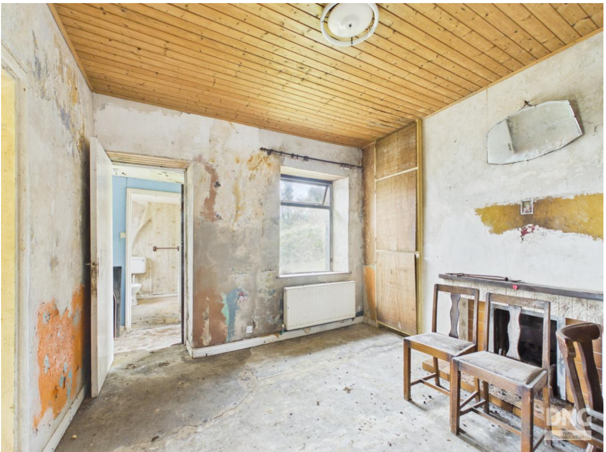
Derelict Residence, Ashbrook, Strokestown, Co. Roscommon
